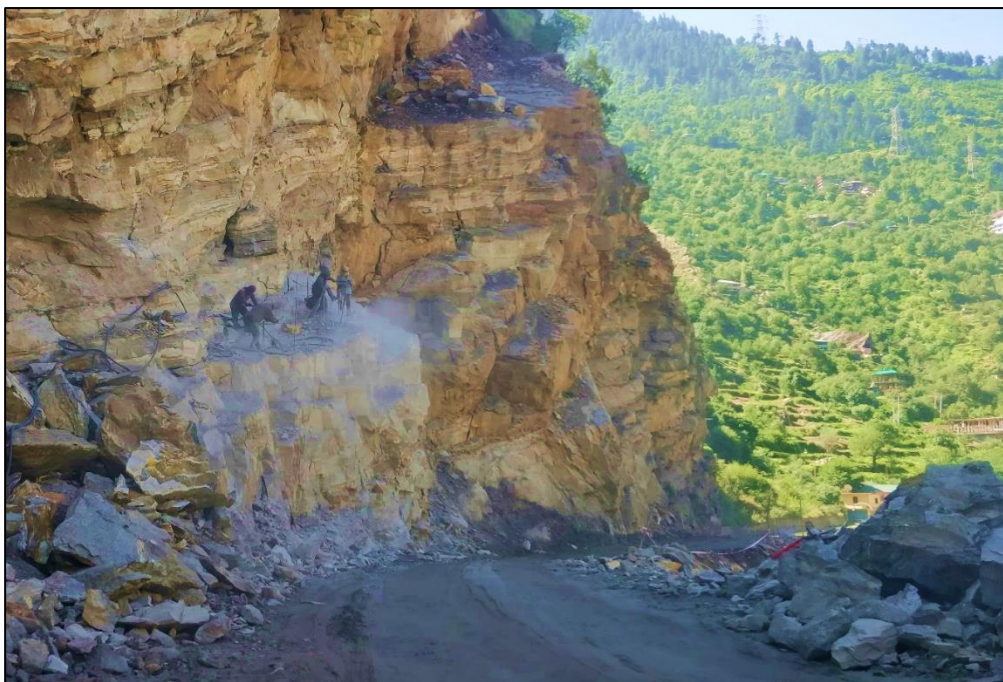
Figure 10. Road widening (Men at work) on NH-5 connect Shimla to Kaza via Kinnaur. Source: Primary Survey, 2017.
