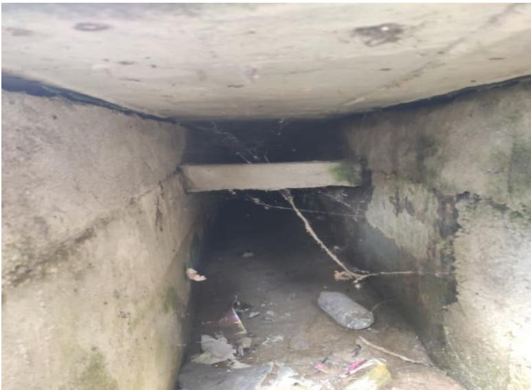
Figure 5: Improper cleaning of storm drains
