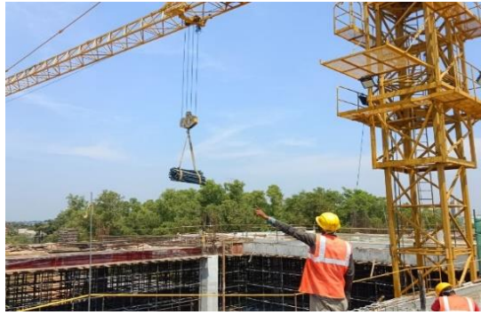
Fig.4 Hand Signal given to the crane operator to swing the boom of the crane
