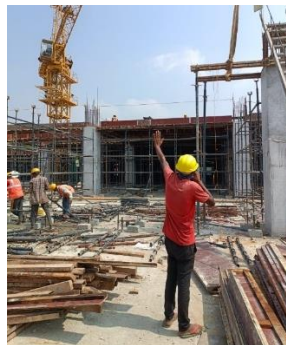
Fig.6 Construction worker giving signals without safety boots
